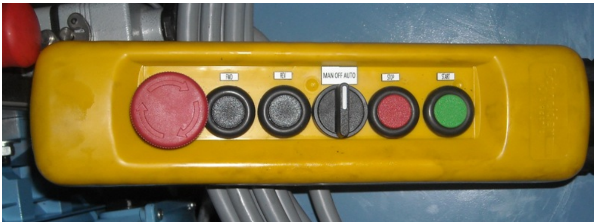
Pulling Gun & Pump Control Buttons
