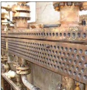
FinFan cooler before a maintenance
